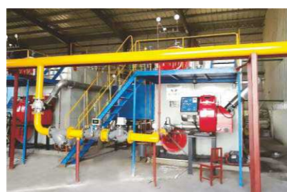
河南郸城薯业公司 10吨低氮冷凝锅炉 10t/h low nitrogen condensing boiler for Henan potato industry
